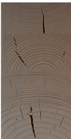
Abb. 8: Schwindrinne in Brettschichholz
