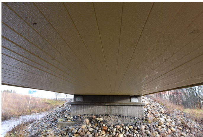
Figure 2. Condensation on bottom of the bridge deck.
