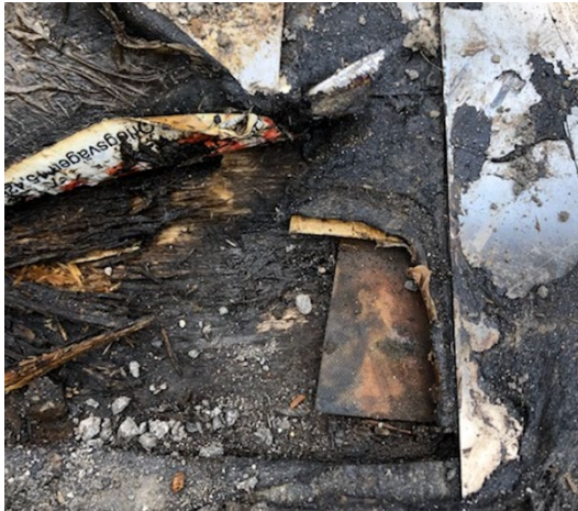
Figure 6. Detail of Gislaved bridge. Membrane strip not properly attached. Decayed wood is also visible.
