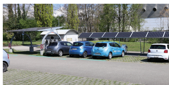
Analyzed PV charging stations and power stations and at Campus Tiergarten in Burgdorf.
