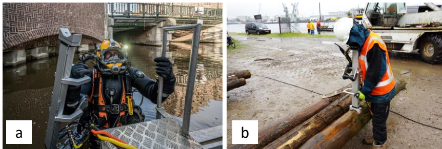
Figure 4: Micro-drilling measurements: a) underwater measurements on wooden piles; b) measurements after piles extraction.
