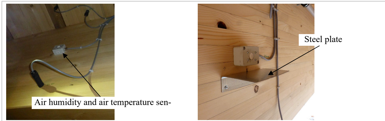
Figure 4 Air humidity and air temperature sensor (left) and steel plate as radiation protection (right).
